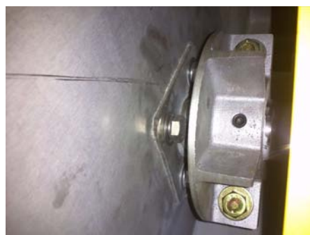
Shaft Cooling Wheel
